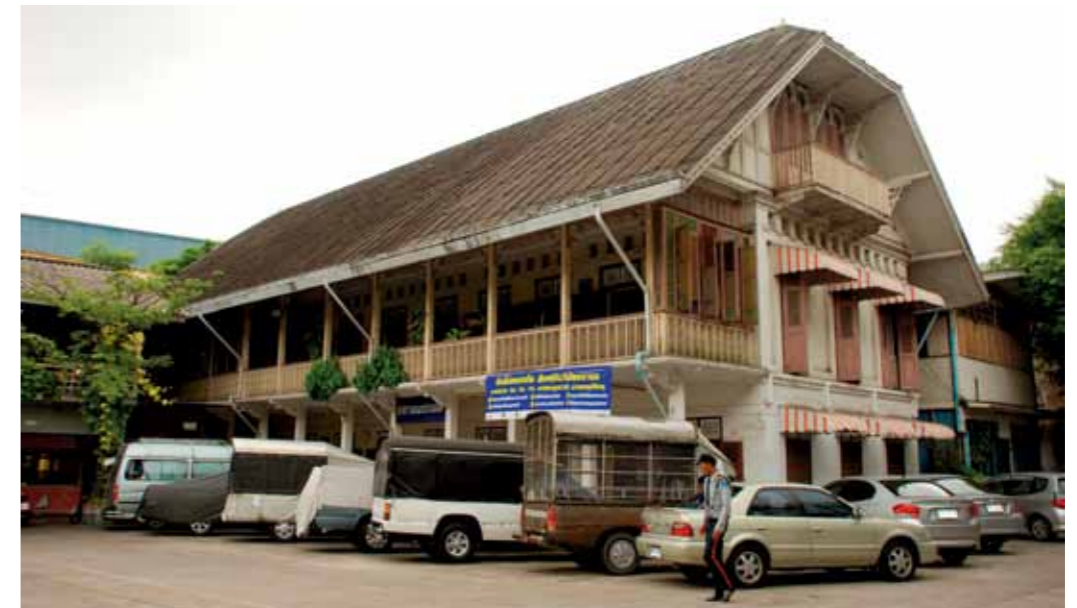
Figure 18. Former residence of Phraya Sri Thammathirat under restoration. The project is funded by the tenant, Sitabut Barmung School and Sino-Thai Foundation for Culture and Education (source: CPB)
